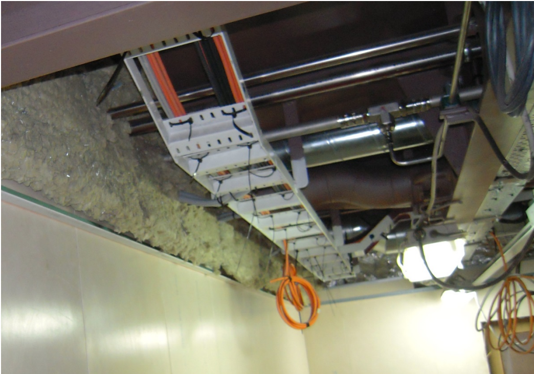
Noise insulation above ceiling - cabin to cabin/corridor.
