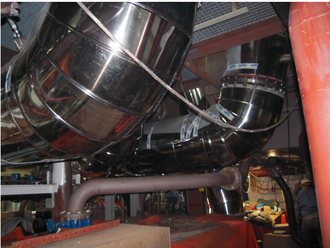
Exhaust pipes encapsulated
